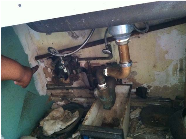
A hole beneath the kitchen sink in Sonja Bent's apartment
